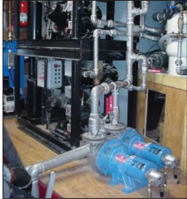
The compression unit and power supply.
