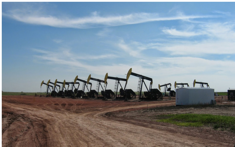
Figure 21. A multi-well pad during production in the Bakken Shale: likely, electrical pumps would be used in Western Newfoundland
