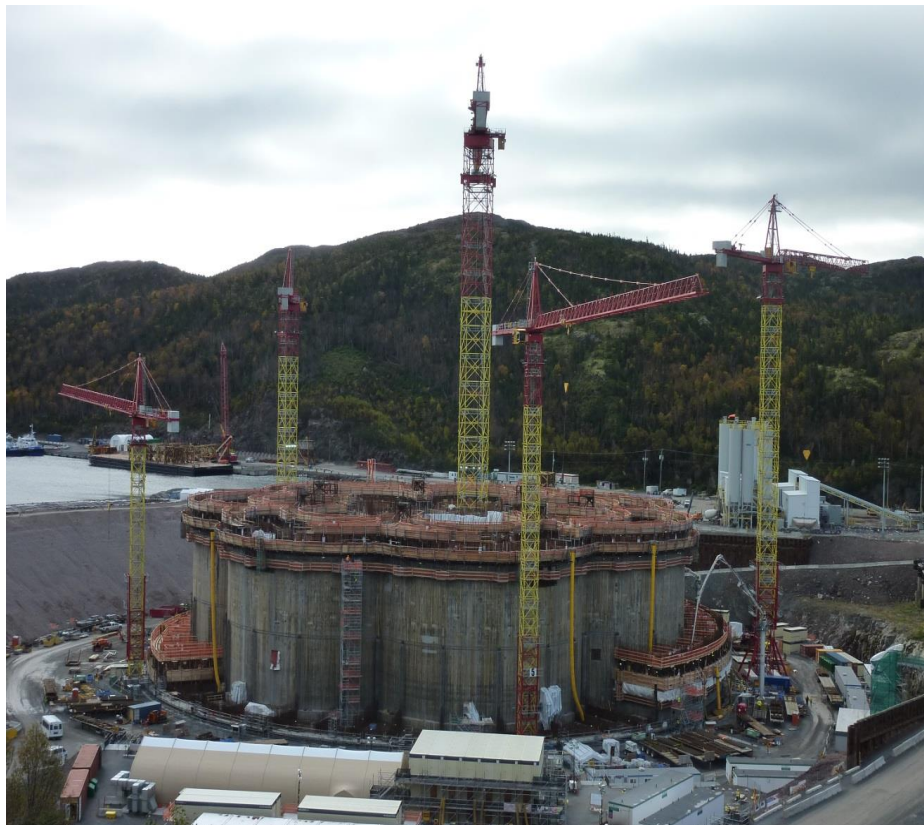
Figure 5. Hebron GBS is being built at the Bull Arm Site in Newfoundland (photo courtesy of Darrell Spurrell, NL DNR).
