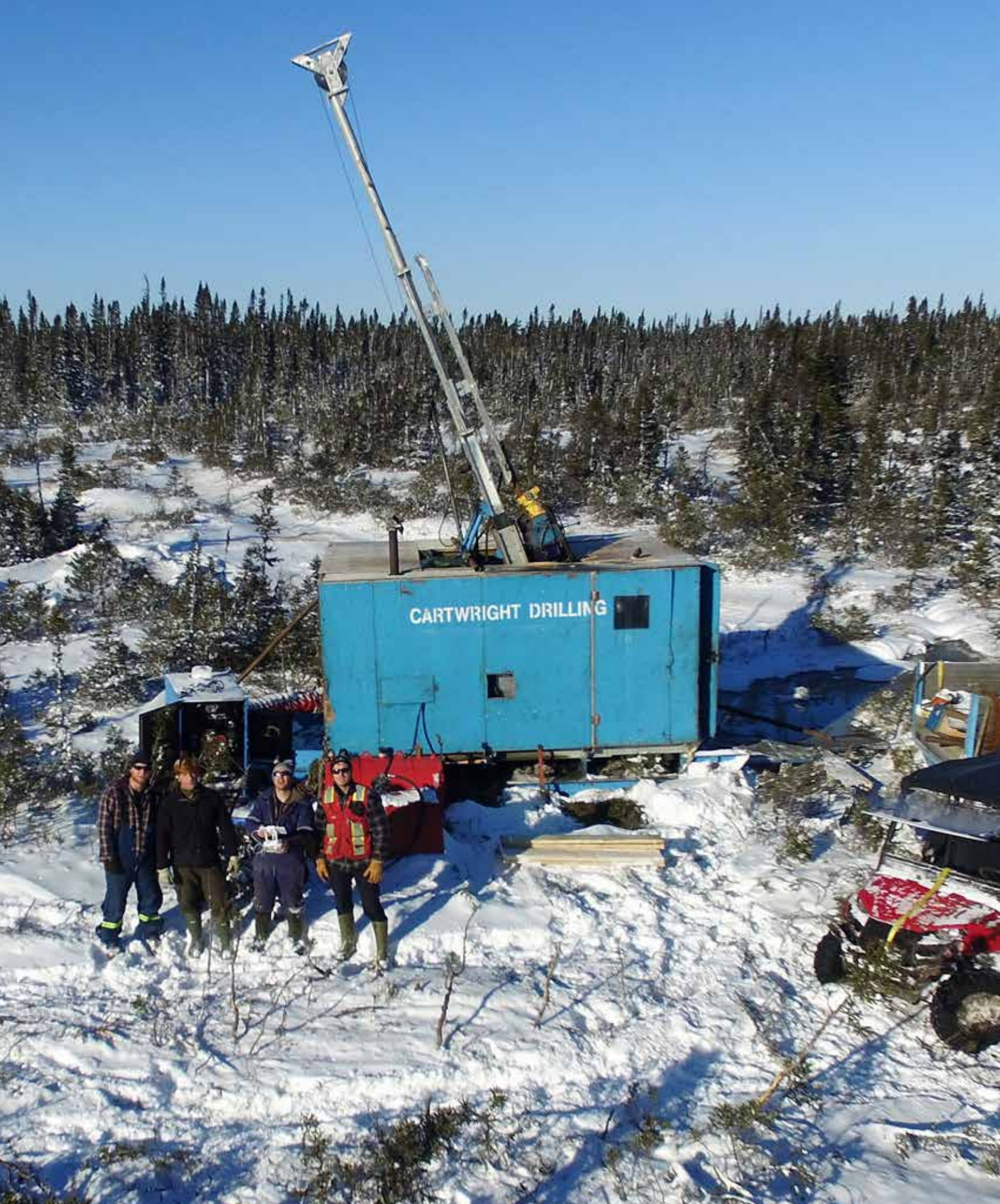
Drill rig and field crew, Lynx Lake copper-cobalt project, King's Bay Resources Corp.
