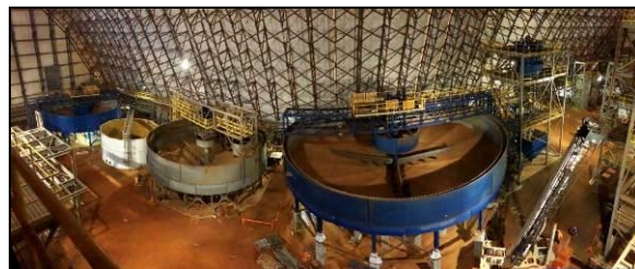
Processing plant dome interior, Timmins site, DSO project, Tata Steel Minerals Canada.
