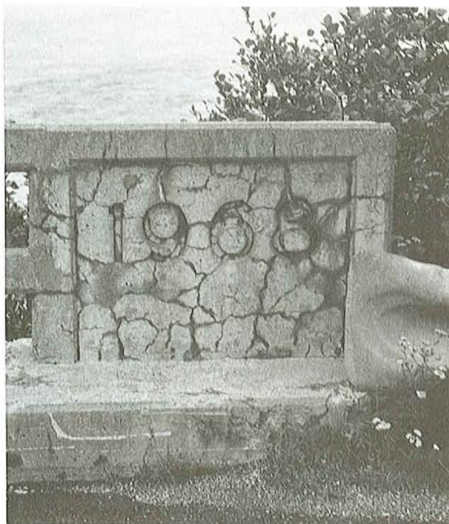
Plate 13. Deterioration due to alkali-reactivity.
