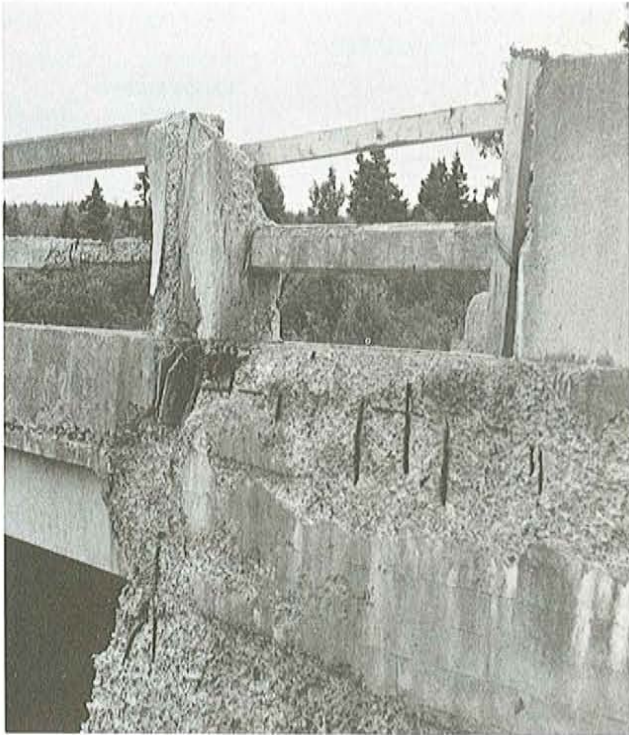
Plate 12. Deterioration due to freeze/thaw.
