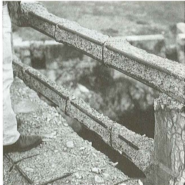
Plate 7. Intensive deterioration in bridge.
