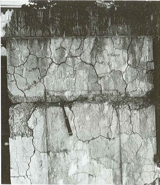
Plate 16. Cracking due to alkali-reactivity.
