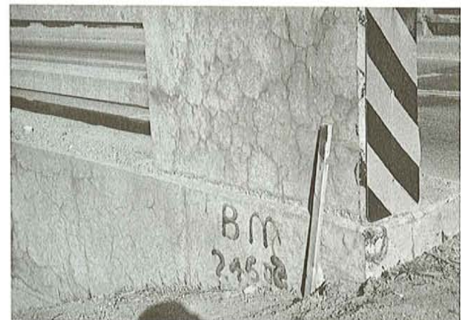
Plate 9. Bridge abutment showing only minor cracking.
