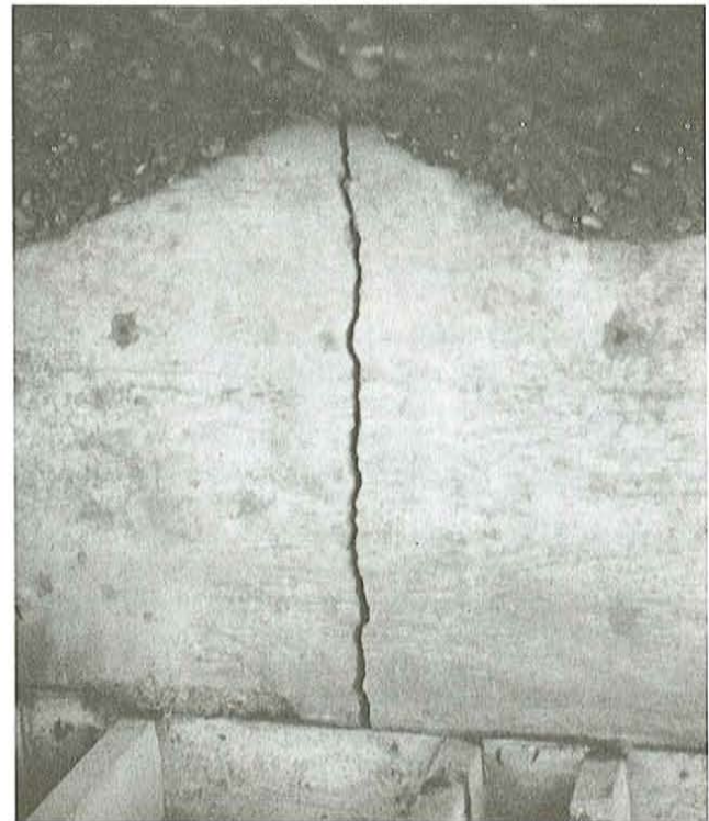
Plate 15. Cracking due to tension.
