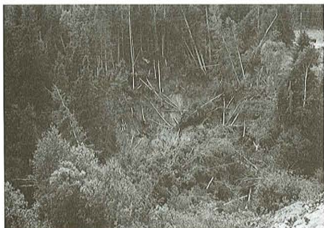
Plate 5. A small landslide opposite the Cormack intersection on the Viking Highway. The slide occurred during heavy rains when fluvial sands overlying a compact diamicton became saturated and failed along the contact.
