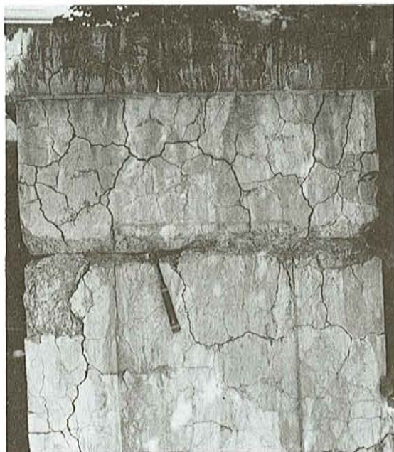
Plate 2. Premature deterioration of concrete, showing pattern cracking due to alkali-aggregate reactivity.
