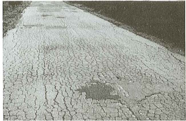
Plate 3. Premature deterioration of asphalt, caused by poor aggregate being used and poor design.
