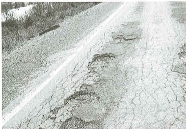
Plate 3. Premature deterioration of asphalt pavement, Bay d'Espoir Highway, Newfoundland.
