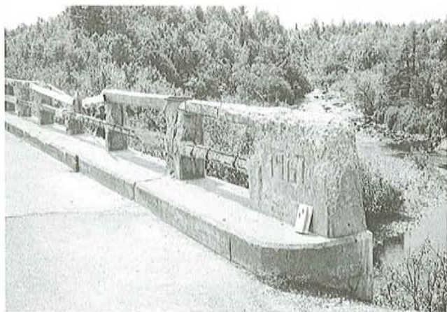
Plate 4. Premature deterioration of concrete bridge, Norris Arm, central Newfoundland.
