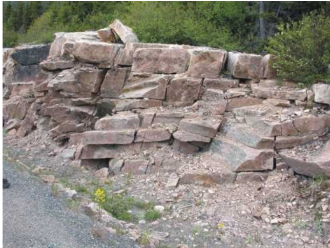
Plate 12a. Orthogonally jointed Dunamagon Granite in a rock cut along the Pacquet road, 2 km northwest of Woodstock.
