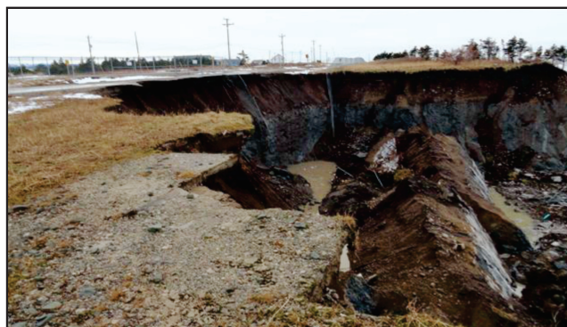
Plate 2. In November 2013, a large amount of sediment was displaced in Daniel's Harbour during a landslide, damaging part of the old roadway that was closed in 2007 due to a previous landslide in the area.
