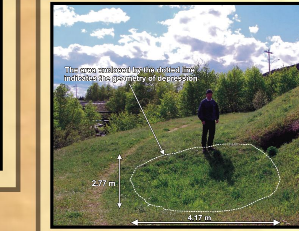
View of the surface deformation and depression
