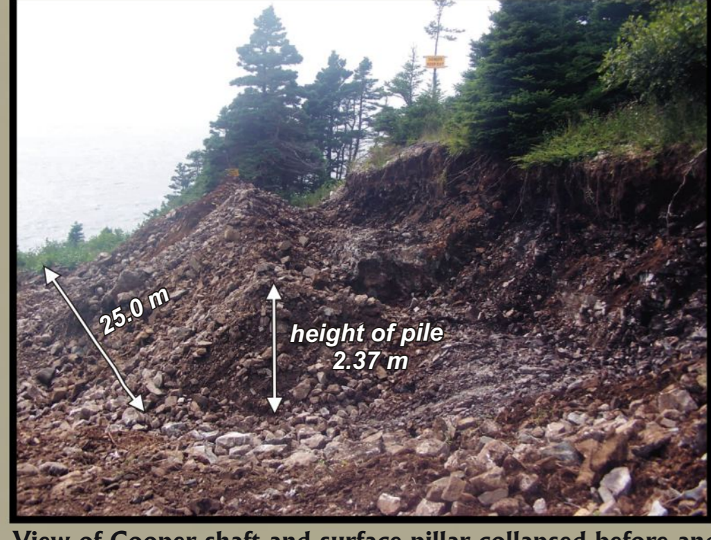
View of Cooper shaft and surface pillar collapsed before and after rehabilitation
