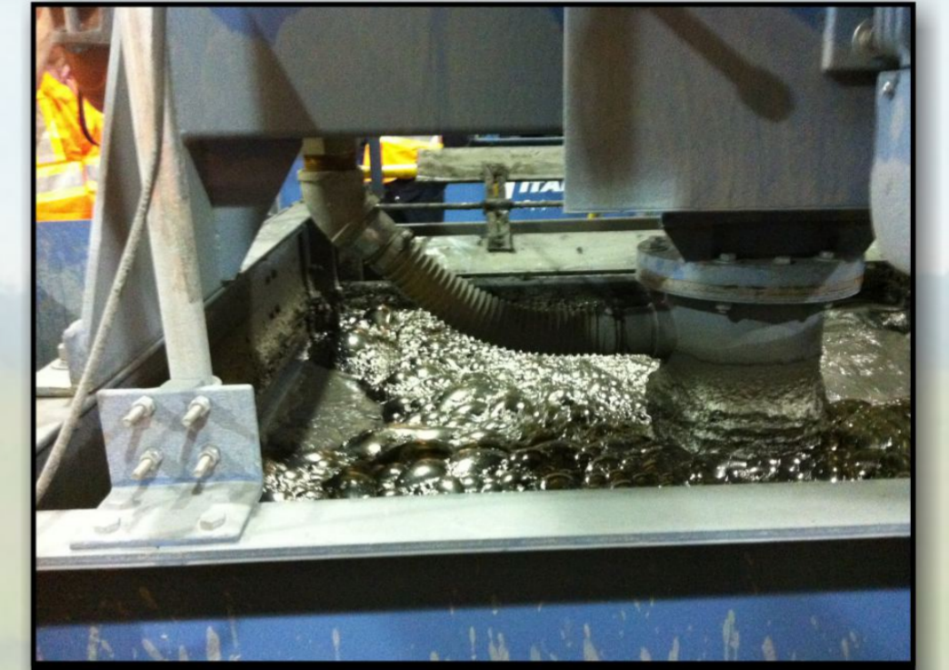
Rambler Metals and Mining – New Copper Mill Commissioned June 2012
