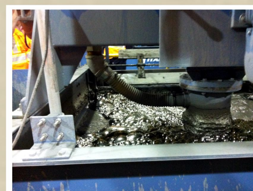
Rambler Metals and Mining Canada Limited commissioning its new copper mill at Nugget Pond.
