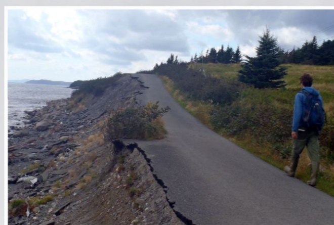
Coastal erosion undercutting a road in O'Donnells.
