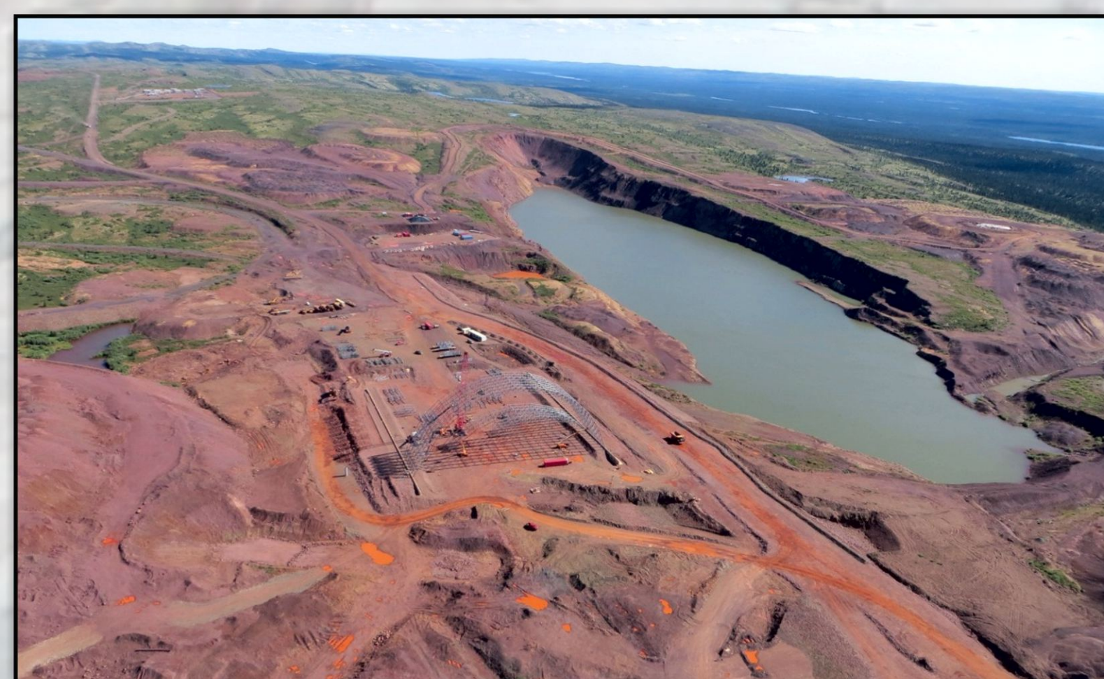
Aerial view of the Timmins No. 1 pit (IOC, exhausted) and construction of Tata Steel Minerals Canada processing facility.
