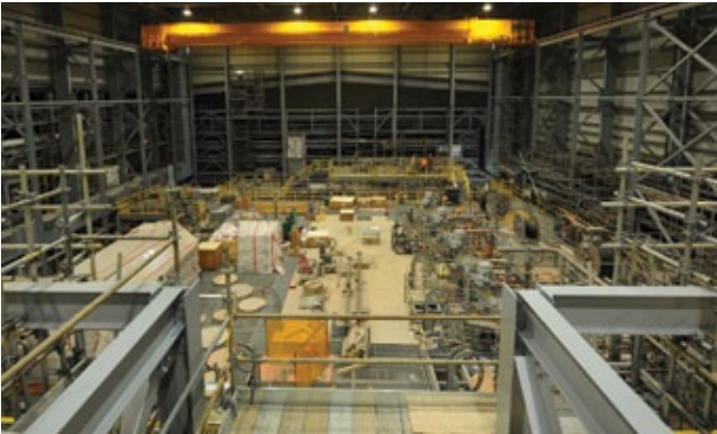
Pressure oxidation leach (POL) building under construction at the Long Harbour processing plant. Photo courtesy of Vale.
