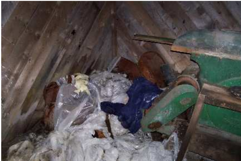
Photo 27: Deteriorated Drums inside Storage Shed. (Note the Discarded HazMat Suit)
