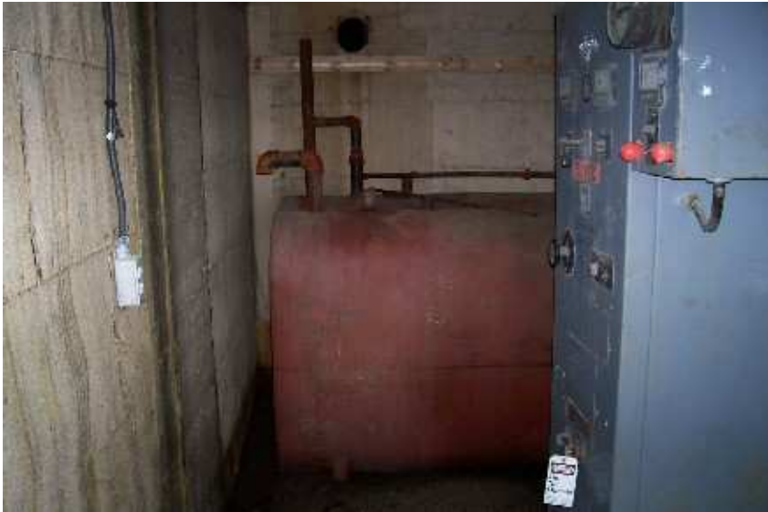
Photo 1: Two 200-Gallon ASTs - Main Mill Generator Room. (Rambler Main Mine)
