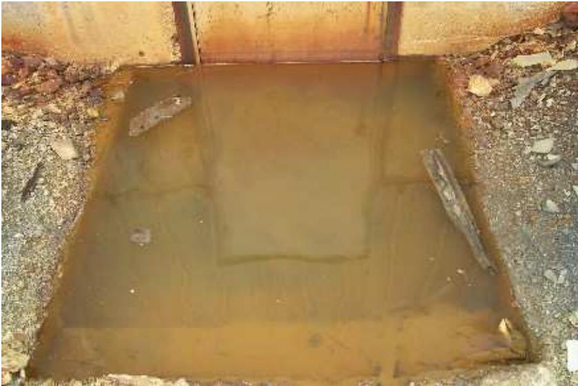
Photo 33: Flooded Rear Entrance to Maintenance Garage.
