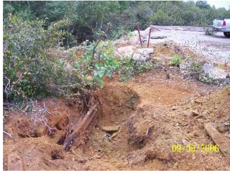
Photo 14: Potential Air and Wire Pipelines – Building No.3. (Not UST Fill and Vent Pipes)
