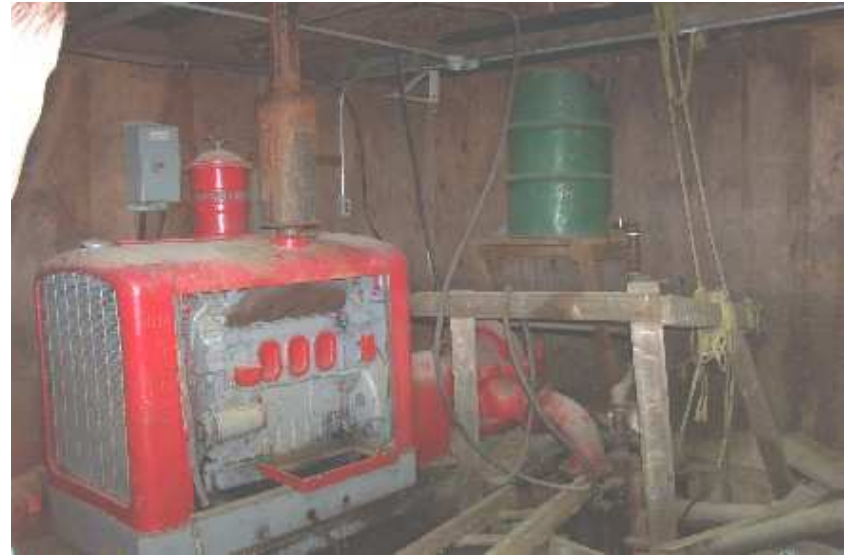
Photo 18: Pumphouse – Diesel Powered Pump.
