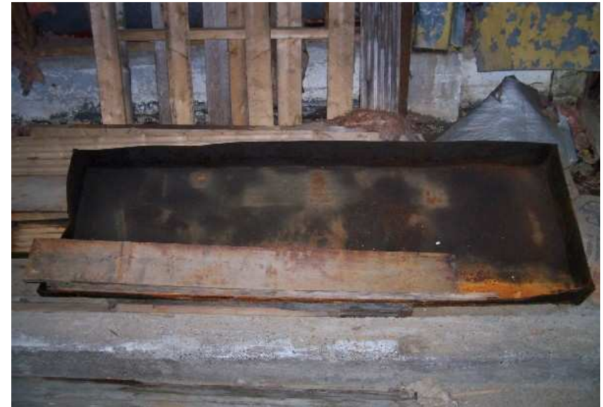
Photo 12: Oily Metal Pan - PCB Storage Area of Building No.2.
