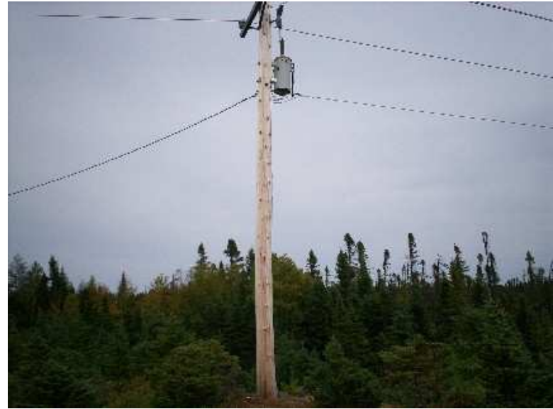
Photo 10: Pole-Mounted Transformer Along Hydro Cut-Lines.
