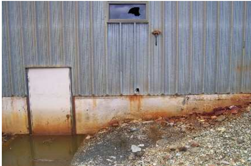
Photo 31: Stain Area at Rear of Maintenance Garage. (Note Hole in Siding – Possible Fuel Line Hole)
