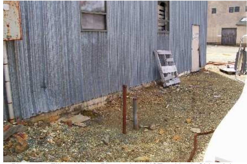
Photo 30: Fill and Vent Pipes of an UST at North Side of the Maintenance Garage.
