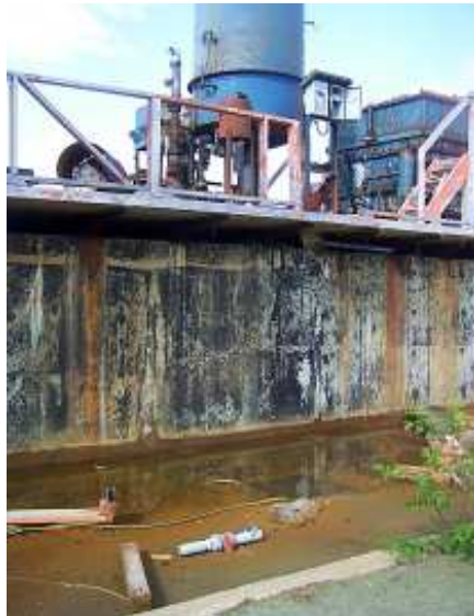
Photo 7: Possible Sump – North Side of the Facility.
