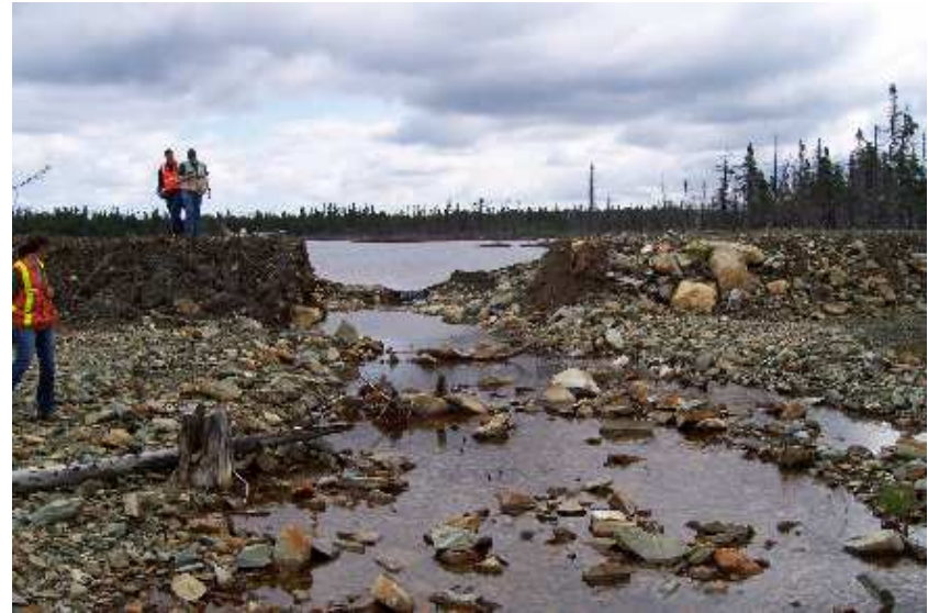
Photo 6: Collapsed Section of the Dyke/Bern between Muskrat Pond and the Tailings (i.e. Breach).
