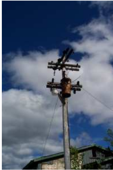
Photo 5: Transformer #1. (West of Bunkhouse No.2)
