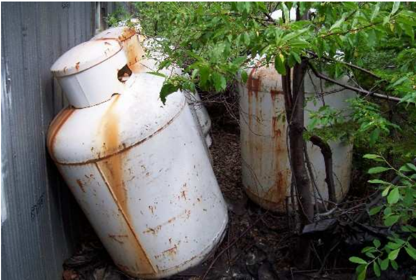
Photo 11: Four Propane Tanks. (Southside of Bunkhouse No.2)
