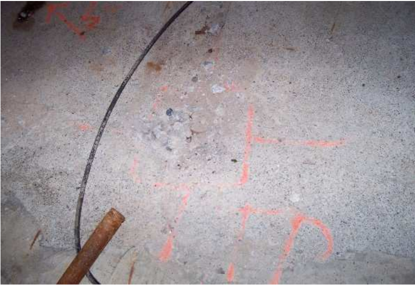
Photo 13: Building No. 2 - PCB Storage Area. (Location of JWEL TP-1: PCB 130 mg/kg)
