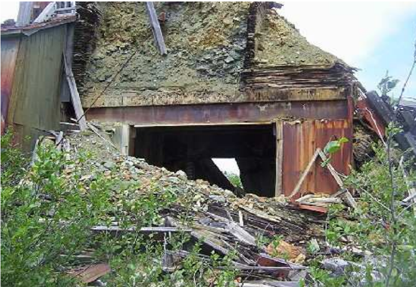
Photo 11: Condition of Building No. 1. (Note Ore Storage and Creosote Timber Debris)
