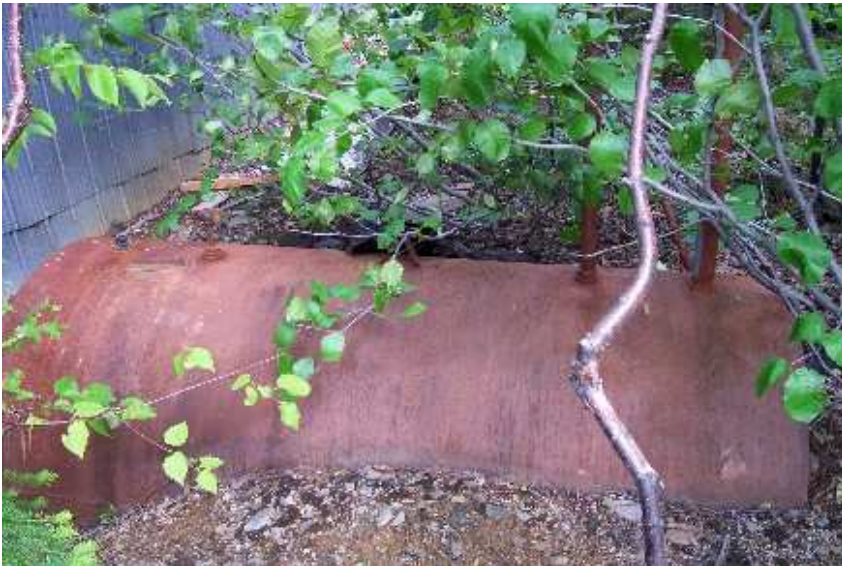
Photo 7: UST Located on Southwest Corner of Bunkhouse No. 2.
