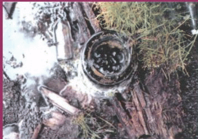
Closeup of intermittent gas bubbles coming from the top of Mills #1 pipe.
