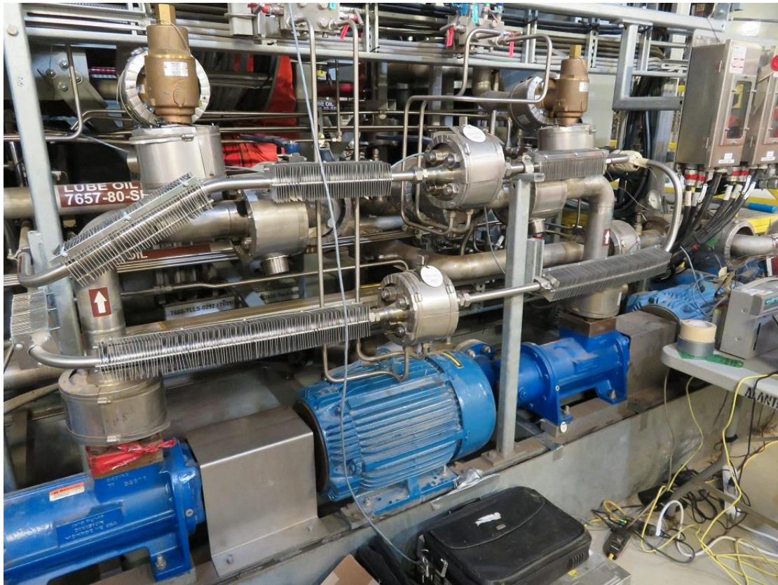
Photo 1: Cooling fins recently added to lubricating oil lines on synchronous condenser, Soldiers Pond.
