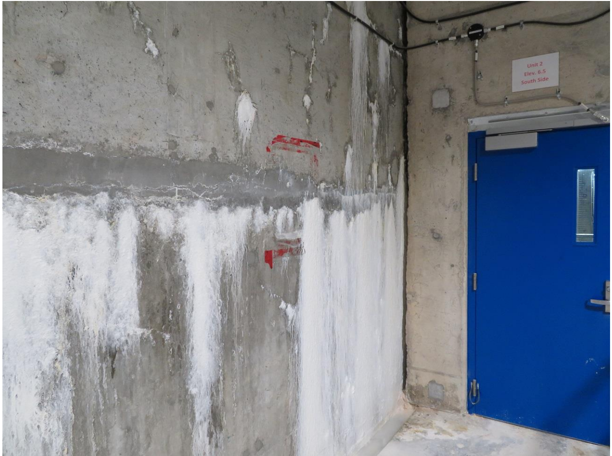
Photo 4: Calcareous material deposited below hairline crack on upstream wall of turbine floor between Units 1 & 2.
