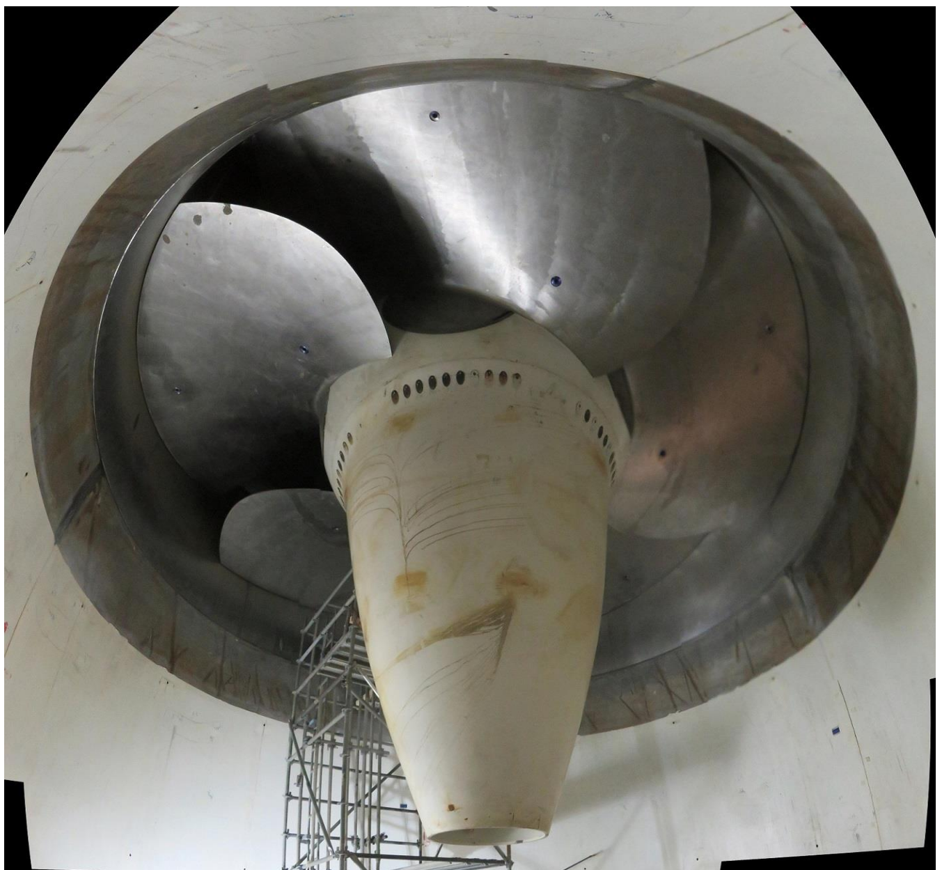
Photo 4: Unit #2 turbine runner viewed from below.
