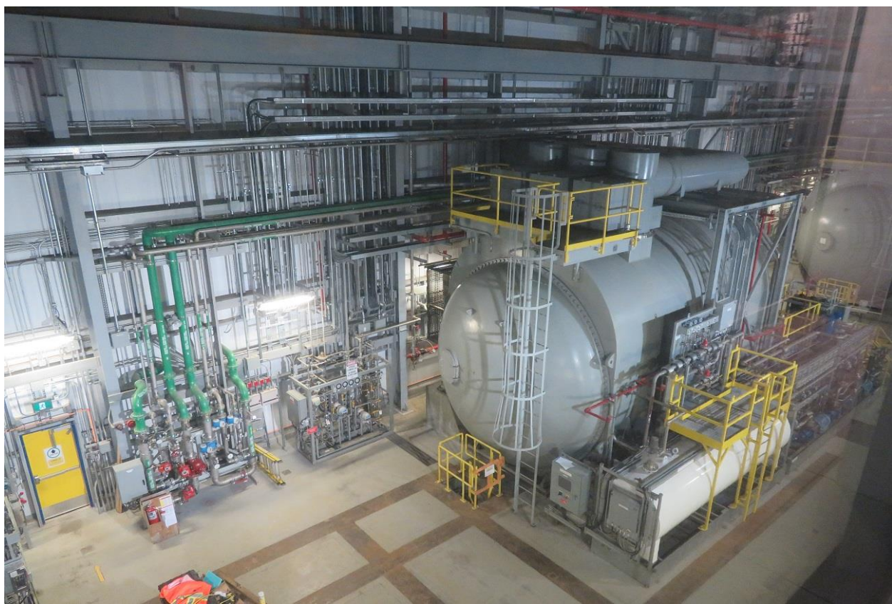
Photo 1: Synchronous condenser, Soldiers Pond.
