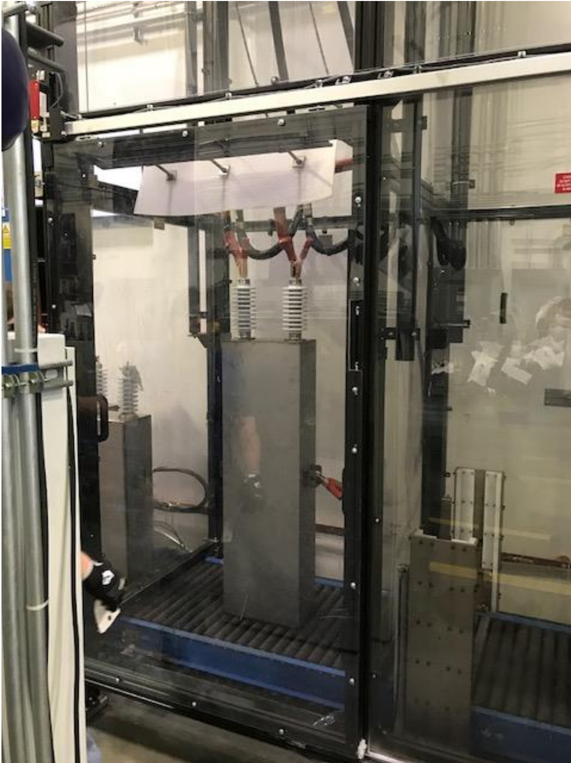
Photo 7: Electrical Test bay.
