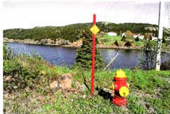
Fire flow water distribution system in Harbour Main.
