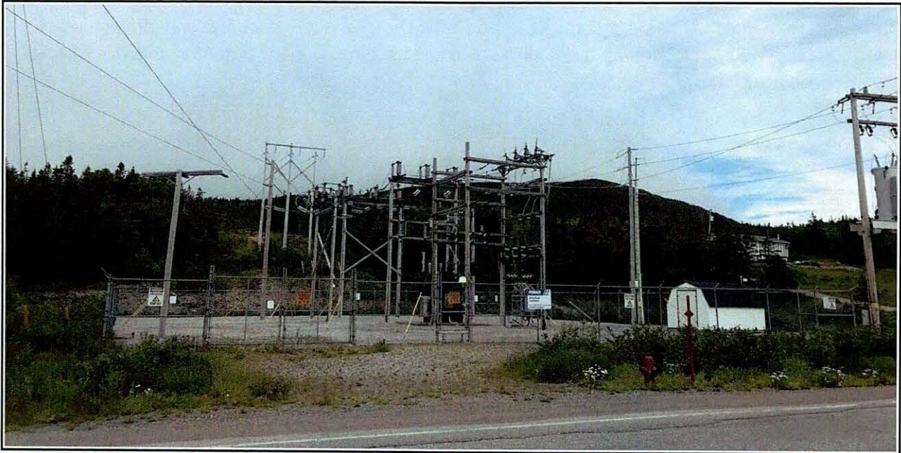
Illustration 9: Public Utility Use, Newfoundland Power Berry Head Substation
