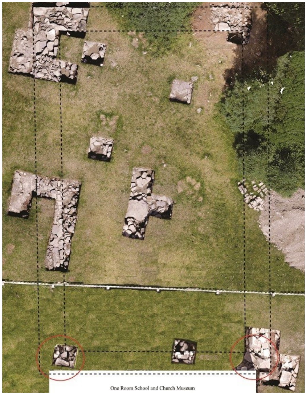
Figure 1: Areas where stones were removed with PAO monitoring to allow weeping tile installation (based on Losier 2022).
