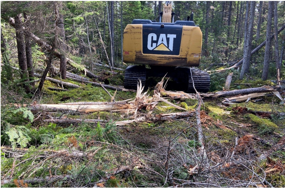
Figure 9: Heavy excavator knocking down trees for access way for geotechnical drilling rig across Sheshatshit high terraces in July 2022.
