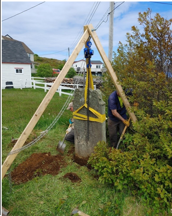
Figure 3: The Hay gravestone, commemorating multiple people who were lost in a house fire, being raised for resetting to level with a chain hoist. Ian Morris (left) and Ian Petty (right) and pictured.
