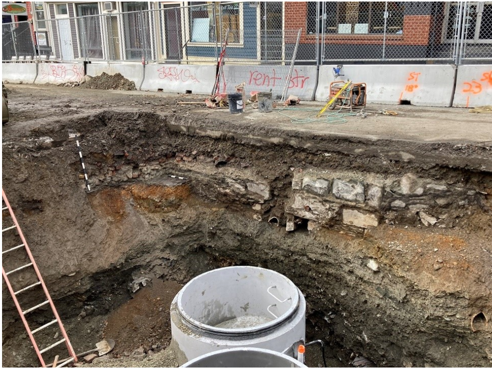
View of the structural features, Duckworth Street, with traces of the wooden “platform” at right (under the photo scales). This wood feature was found to extend out from the wall c. 4.7 m.
