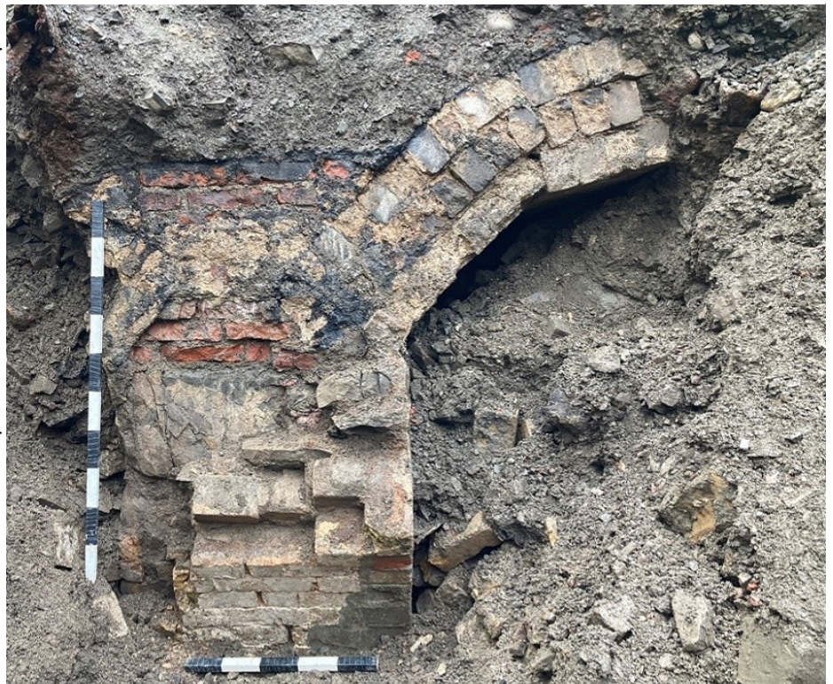
View of an arched foundation feature. Note the brick vaulting extending in two, possibly three, directions.
