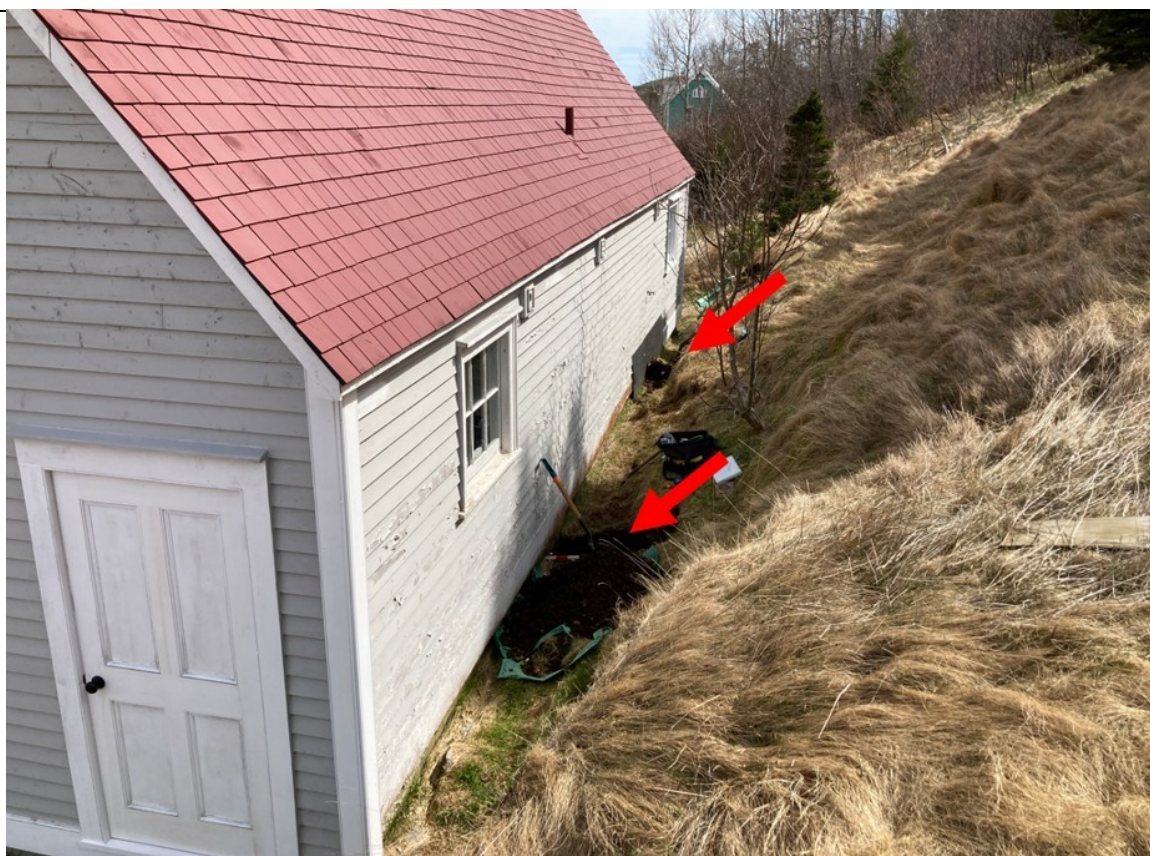
25.02 Figure 2: View of the rear of the Mercantile Premises' modern addition, showing the location of Trench #1 and #2 (rear and foreground arrows, respectively). The proximity of bedrock to the structure is clear.
