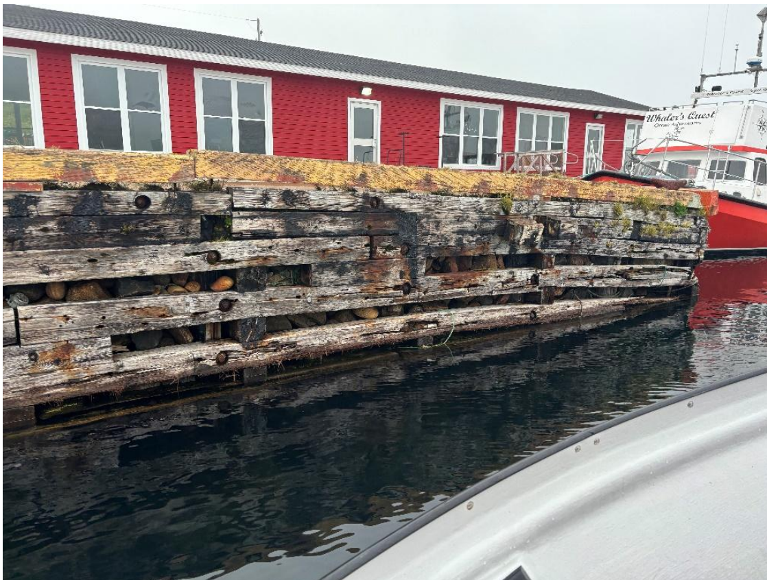
Figure 6 – Dropped southwest corner on west berthing face.
