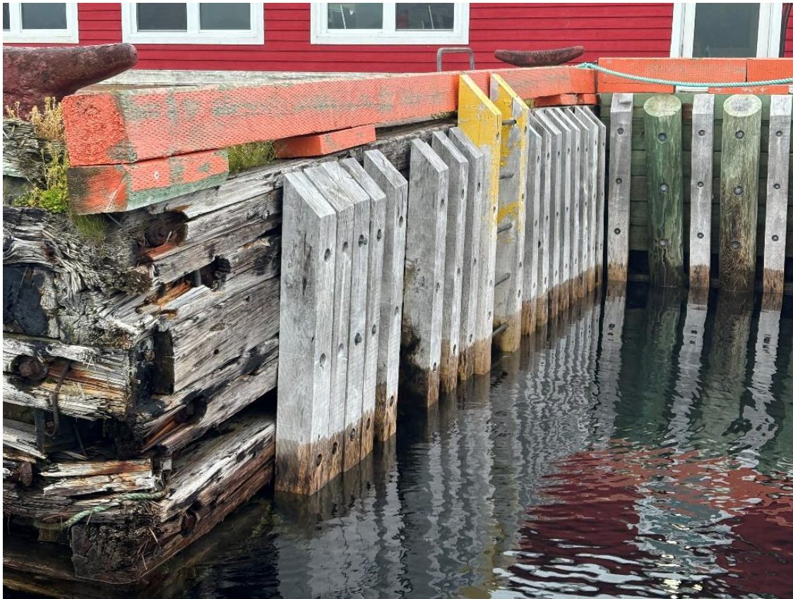
Figure 7 – Damaged timber on southwest corner of west face.
