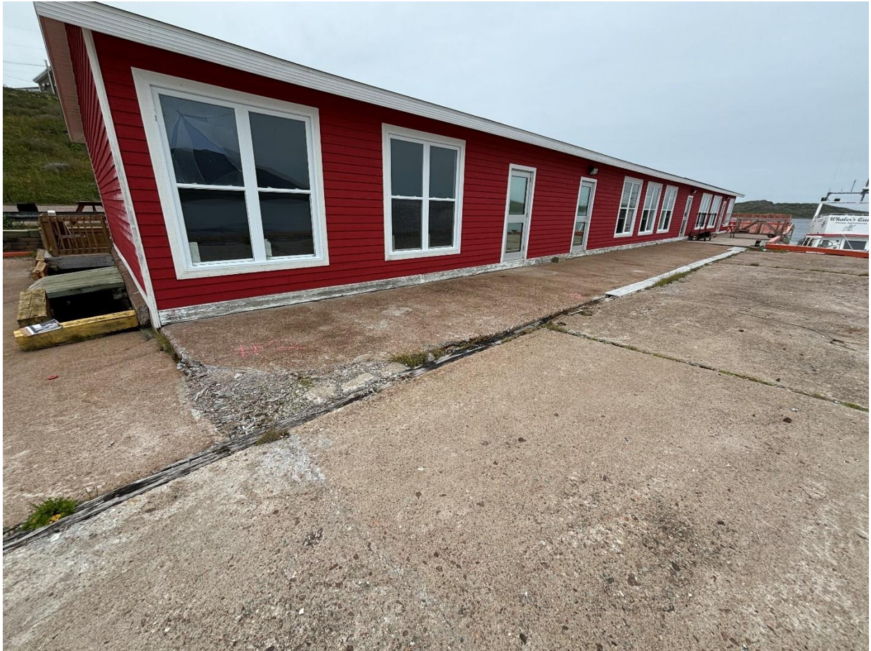
Figure 11 – Building on adjacent wharf with snow fence barrier to prevent access at south end of NL DTI wharf and patio rail to deter access at north end.
