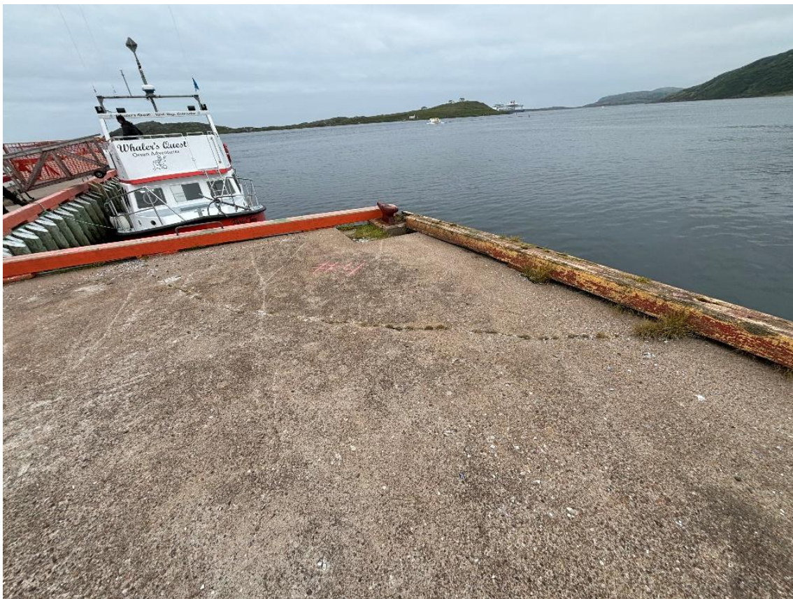
Figure 8 – Wide crack in slab at the dropped southwest corner.
