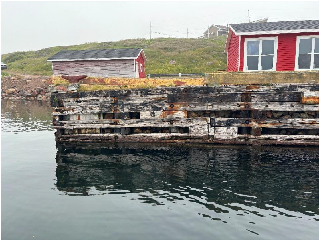
Figure 5 - Dropped northwest corner on west berthing face.
