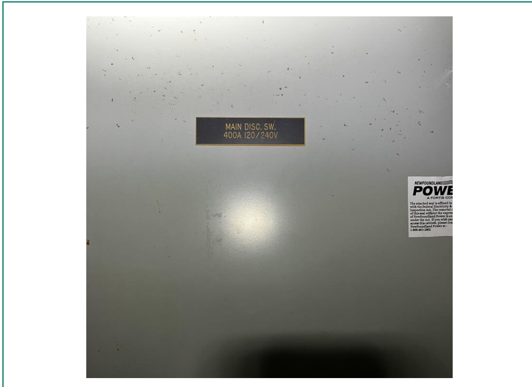
Photo 29: B02 M&E Space - Main Disconnect
