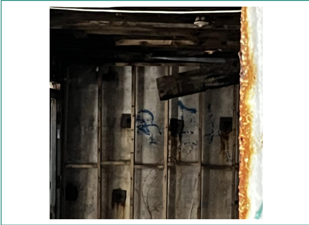
Photo 45: Collapsed Area Level 2 Facing West (Holloway Street)
