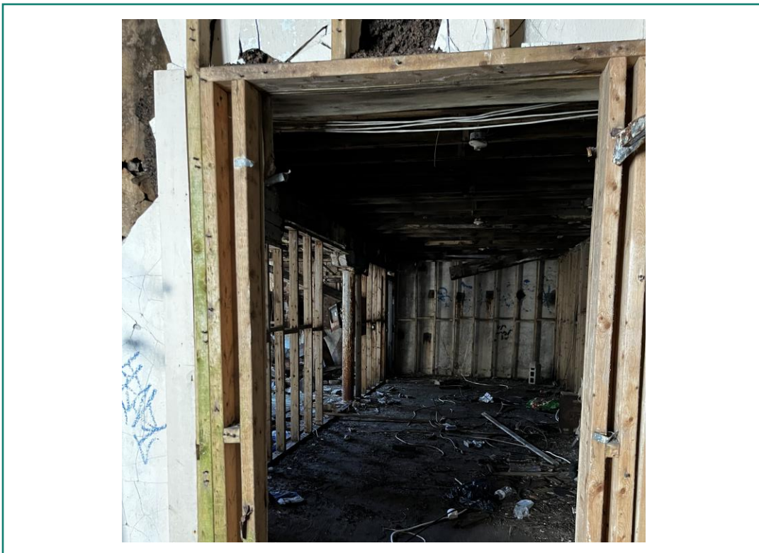
Photo 46: Collapsed Area Level 2 Facing West (Holloway Street)
