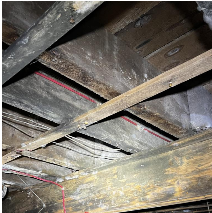
Photo 24: B01 Open Basement Framing
