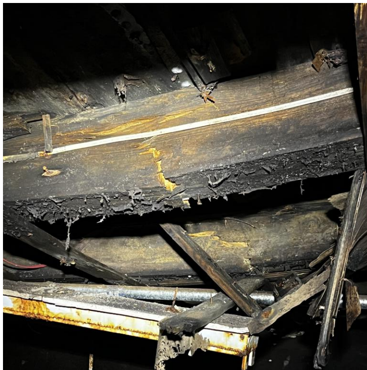
Photo 38: B04 Basement - Cracked Framing Below Tunnel and Corridor
