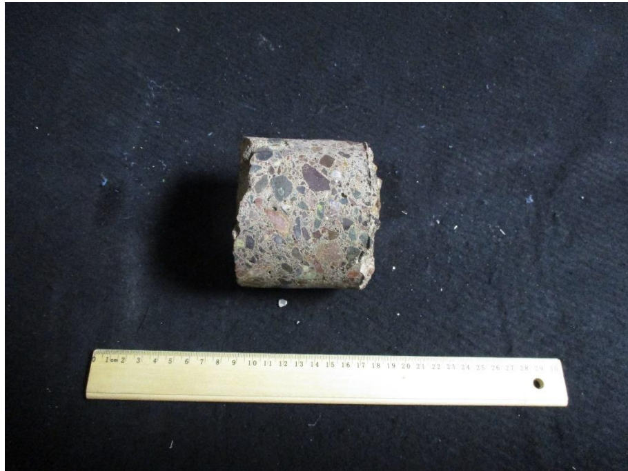
Core D7 Sampled from Bridge Deck
