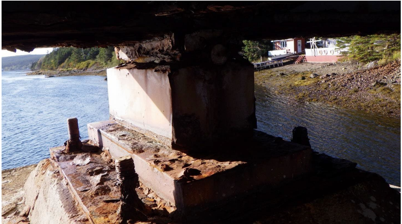
Figure 11. Substantial material loss on bearing components. Pier 1
