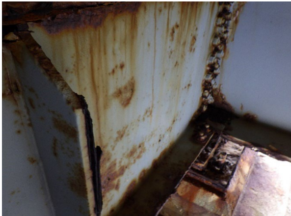
Fig #12 – Rust staining and delamination of coating.
