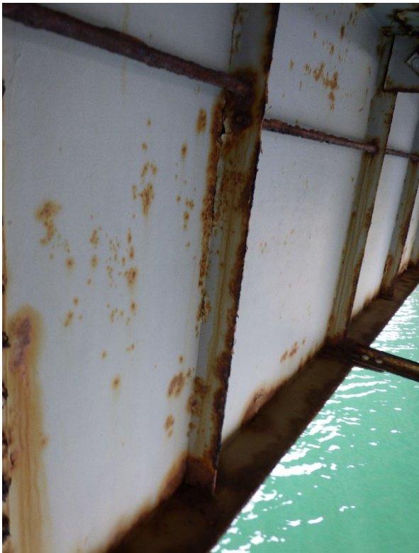
Fig #7 – Typical coating condition on the main bridge beams.
