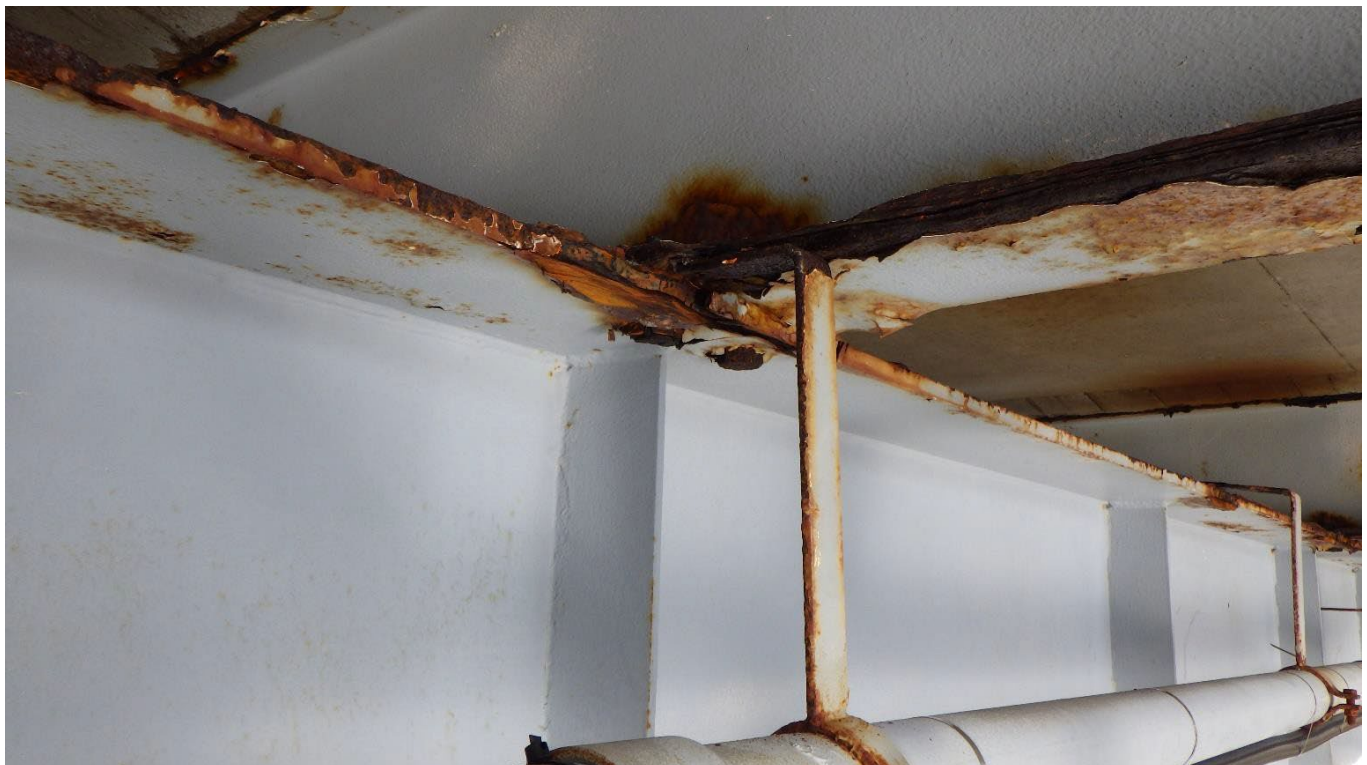
Figure 16. Bracket that has separated from girder.
