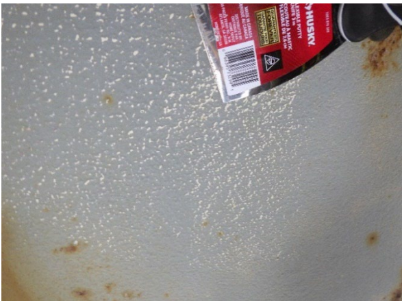
Fig #5 - Scrape test was preformed, showing white layer.
