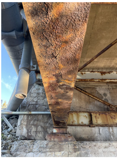
West girder bottom flange looking north. Typical Corrosion
