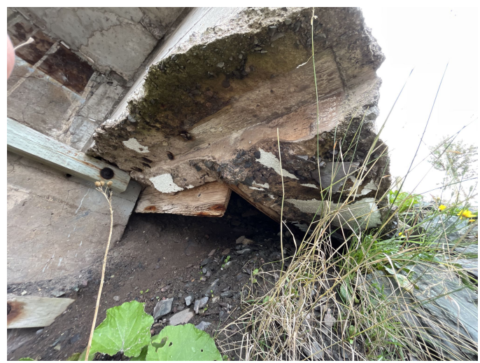
Undermining on Northeast corner extension for sidewalk and end block.
