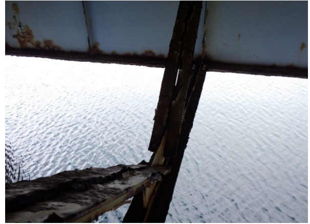
Fig #9 – Typical coating condition on cross bracing.
