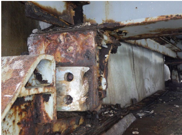
Fig #24 – Coating failure, blistering and delamination.
