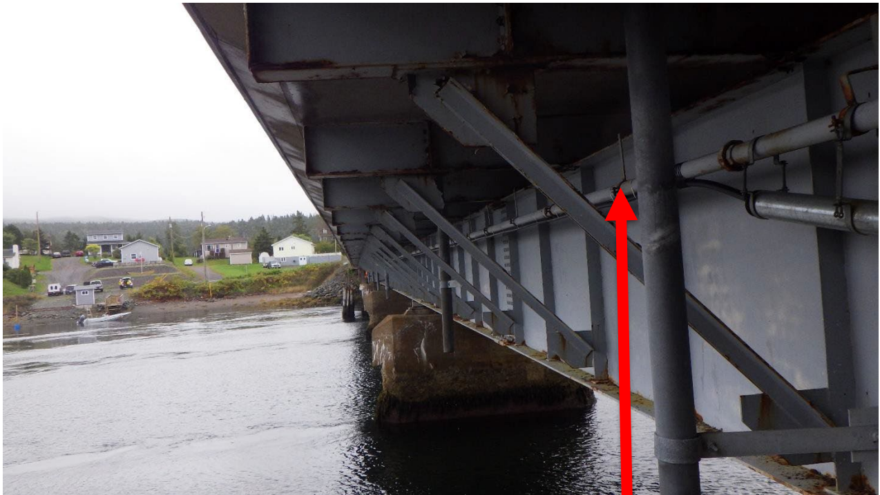
Figure 13. Majority of brackets holding up 4" line is completely detached from girder.
