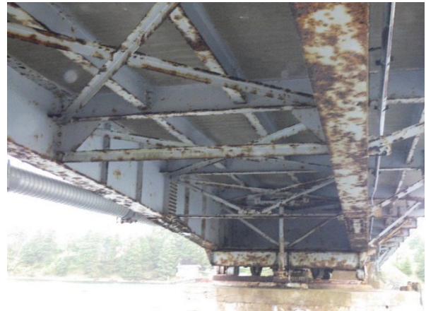
Fig #25 – Rust staining and blistering of coating.
