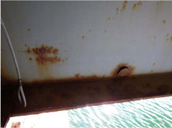
Fig #6 – Typical coating condition on the main bridge beams.
