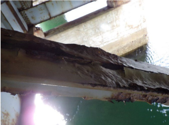
Fig #8 – Typical coating condition on cross bracing.
