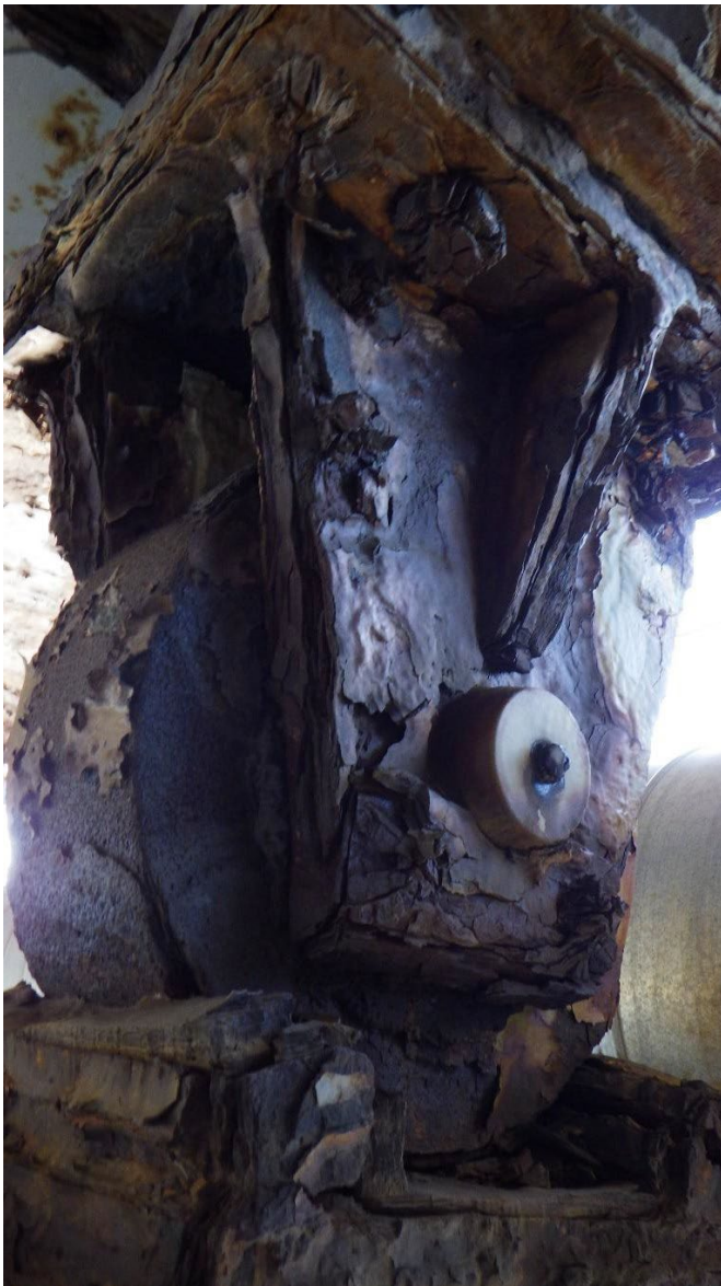
Figure 5. Swing stage pier bearing. Severe corrosion
