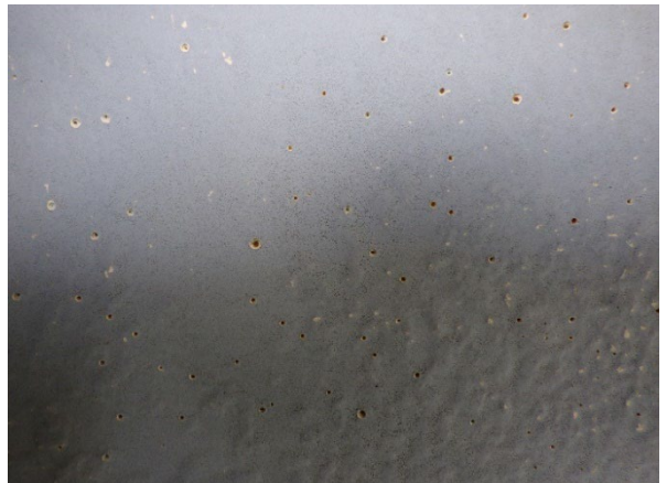
Fig #11 – Rust spots through all coating layers.
