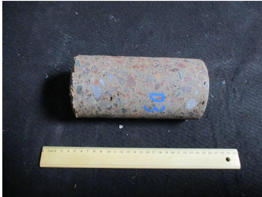
Core D3 Sampled from Bridge Deck
