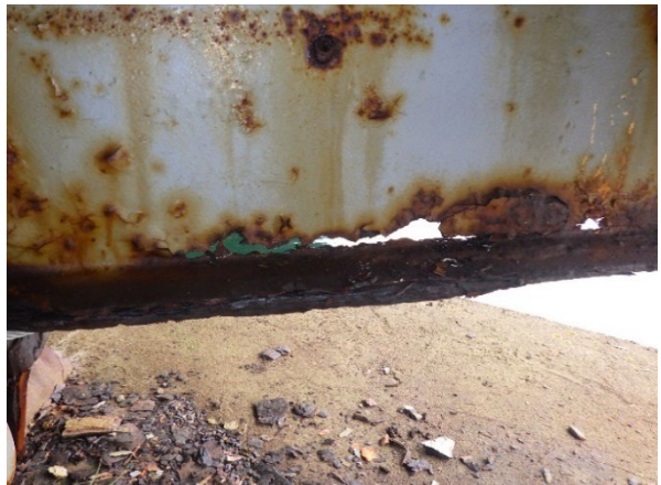
Fig #23 – Hole in swing pier structure.
