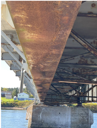
Bottom flange east girder looking south. Typical corrosion.
