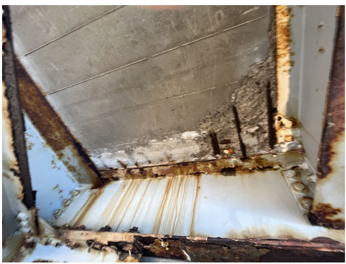
Slab deterioration between east girder and stringer
