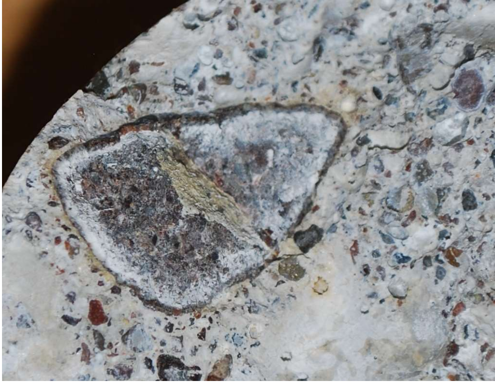
Figure 5: Fracture surface showing dark rim of alkali-silica gel on edge of coarse aggregate particle with white soft AS reaction product in interior of fracture surface through the particle. Field of view = 35mm.
