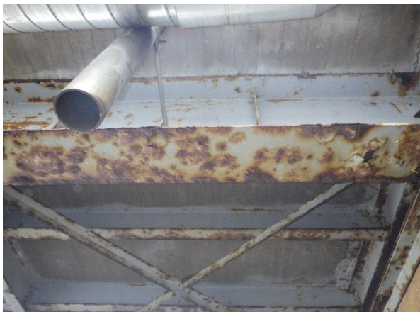
Fig #26 – Main beams, rust staining and blistering.
