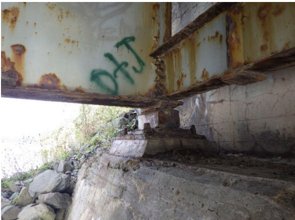
Fig #1 - Example of Blistering, Staining, undercutting.
