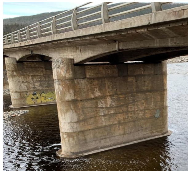
Figure 9-2 – Condition of rounded bullnose on existing pier in service for over 50 years
