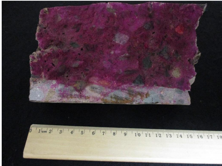
Core D5 – Carbonation Depth Sampled from Bridge Deck
