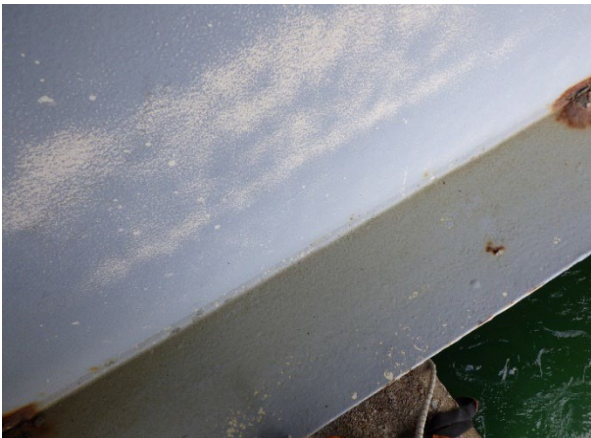
Fig #10 – White coating showing through the topcoat.
