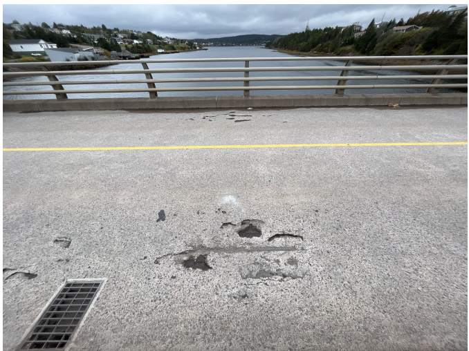
Deck core 3 and defects post 21
