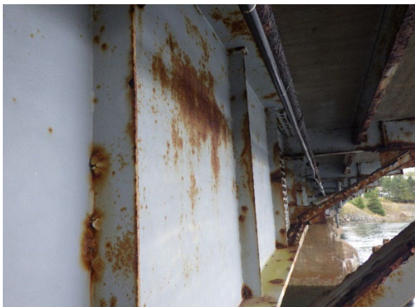
Fig #18 – Typical main beam coating condition.
