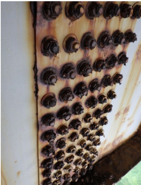
Fig #3 - Corrosion on the hardware of the splice plate
