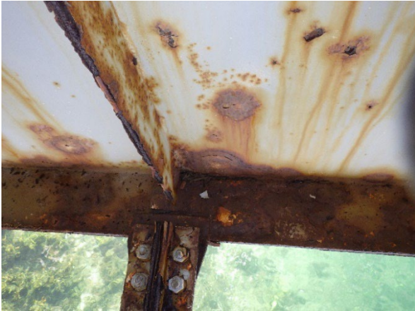
Fig #4 - Typical delamination of the coating from the substrate
