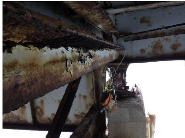
Fig #17 - Swing Pier angle steel, delamination of coating.
