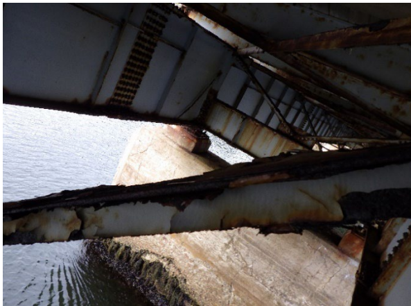
Fig #14 - Heavy corrosion shown causing diagonal connection being disconnected from horizontal piece (Fig #15)
