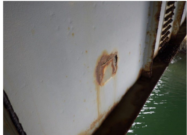
Fig #13 - Example of heat damage, caused by a bracket being welded on the opposite side after initial coating.
