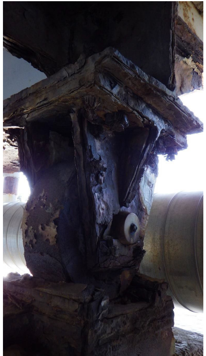
Figure 6. Swing stage pier bearing. Severe corrosion
