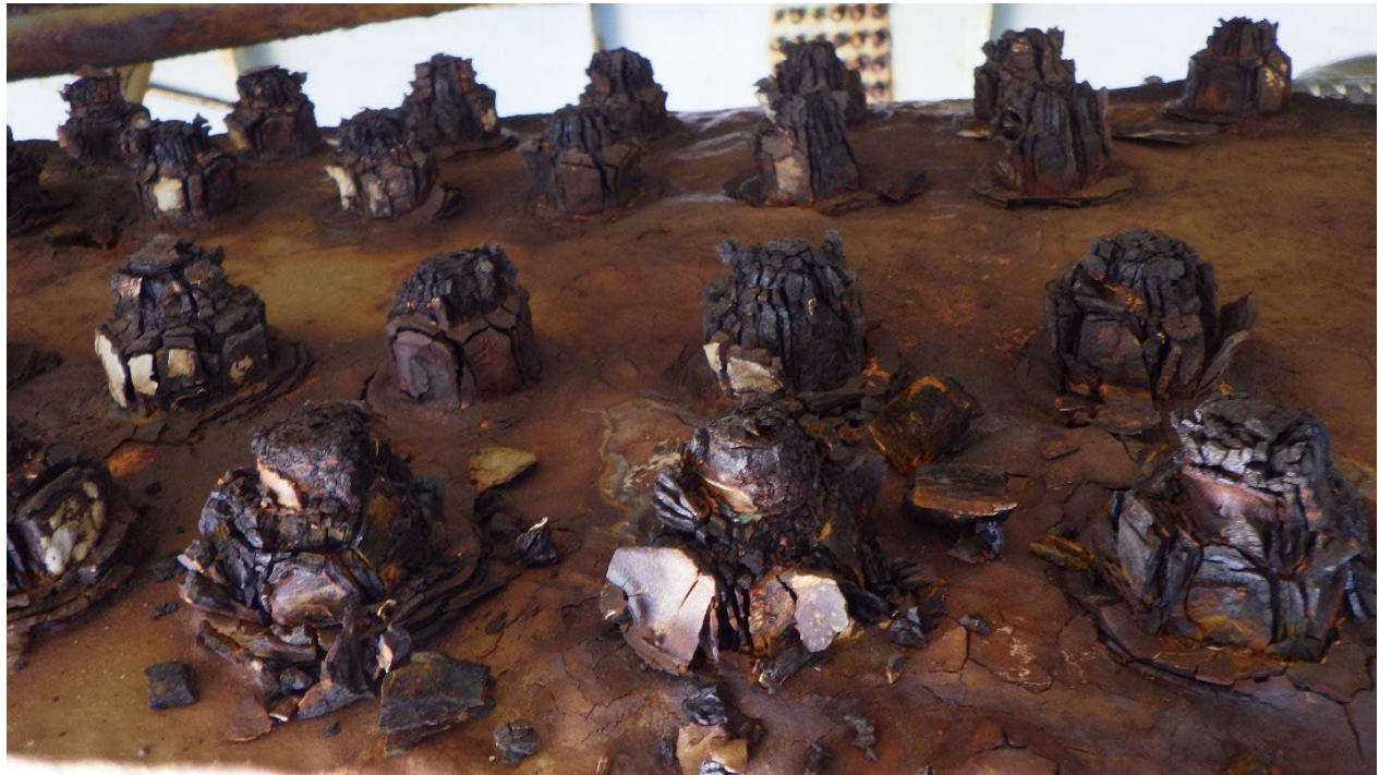
Figure 15. Typical condition of splice plate bolts and nuts, throughout whole bridge.
