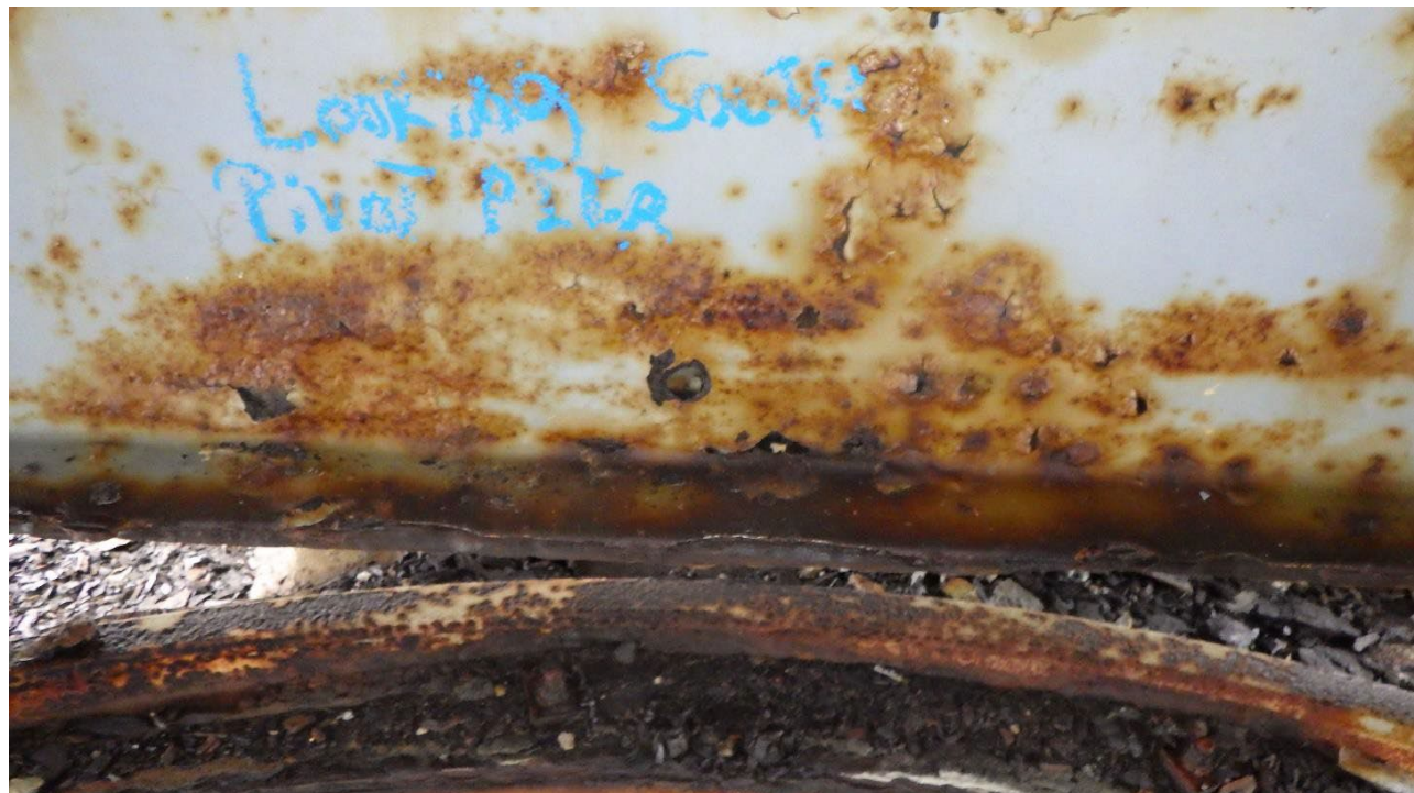
Figure 12. Holes in lateral beam on swing pier.
