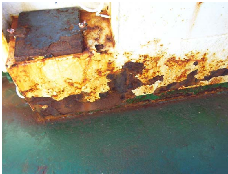
Figure 2.3: Hamilton Sound – Deck Corrosion
