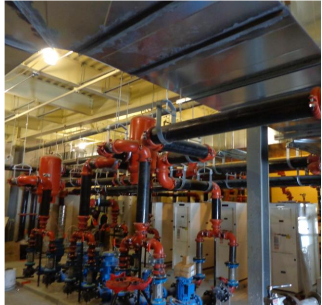
Geothermal Cooling Tower – New Davis Elementary
