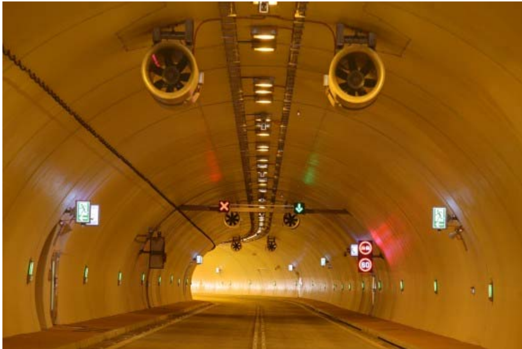
Figure 7-10: Example of Jet Fans installed in a Road Tunnel
