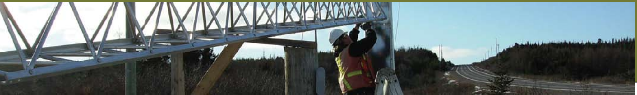
Intelligent Transportation System - Grand Bank Installation
